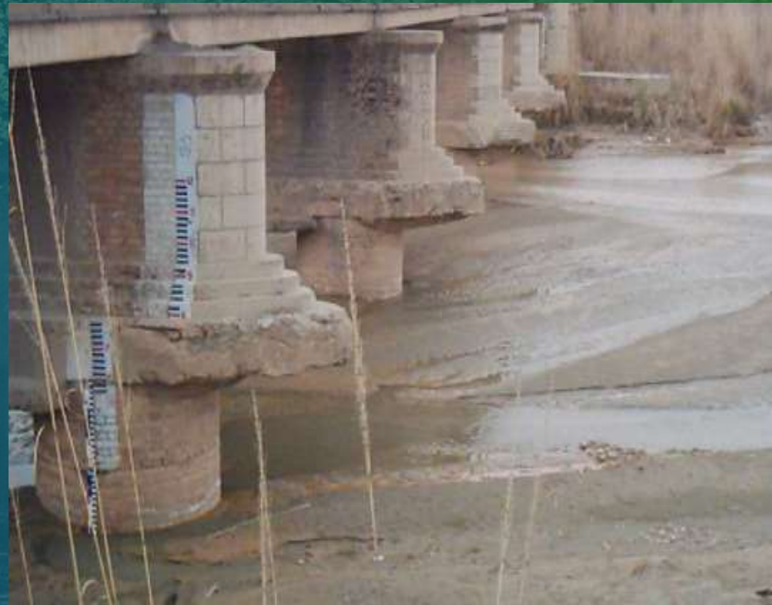
Scouring of foundation
