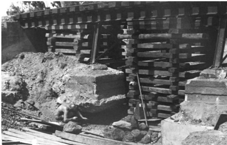
Underpinning the foundations of a railway bridge using a timber box crib to support the bridge. A completed concrete pad underpinning can be seen at the bottom right.]
