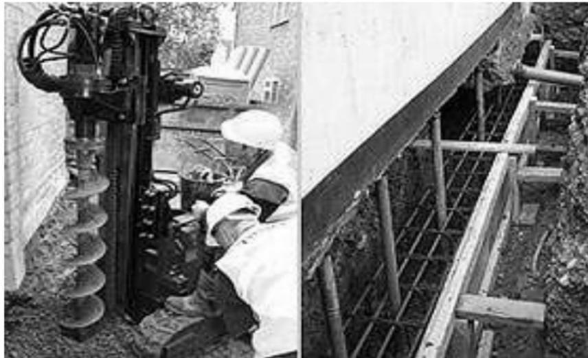
Left: Mini Piling Auger Rig Right: Beam and Base construction of beam under existing wall
